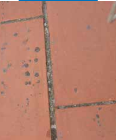
An example of old terracotta floor requiring treatment before applying Aquaflex Roof
