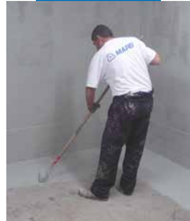
Mapelastic Foundation spread on by roller to waterproof against water in negative pressure
