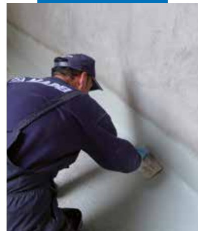
Mapelastic Foundation spread on by trowel to waterproof against water in negative pressure
