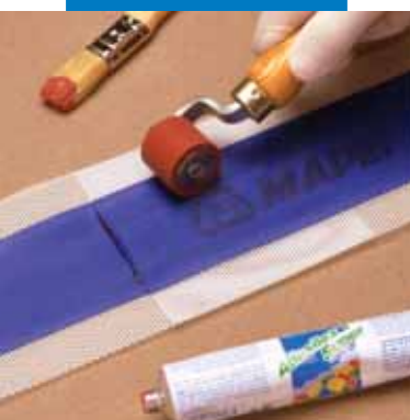
Use a roller to press the joints of the Mapeband strips together
