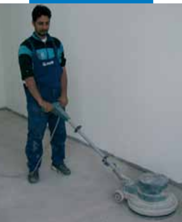
Polishing with helicopter before applying Ultraplan Eco - Mirabello kindergarten - Cantù (Como) - Italy
