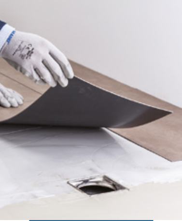
Application of LVT floorings with Ultrabond Eco MS 4 LVT in damp surroundings
