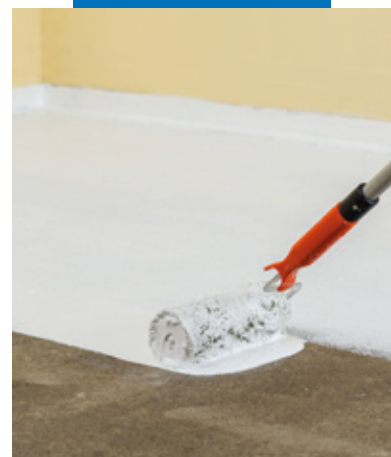
Application of the first coat of Aquaflex Roof Premium on cementitious screed
