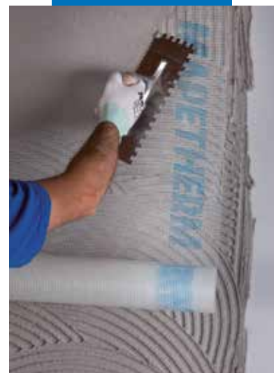
Application of a reinforced smoothing and levelling layer by embedding Mapetherm Net
