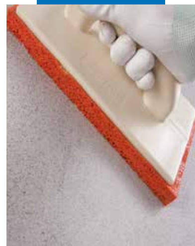
Finishing off the surface of the smoothing and levelling layer with a sponge float
