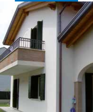
Reggio Emilia - Italy - Work on a private home using Mapetherm AR1 GG
