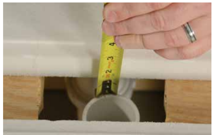
Figure 5: Measure from the top of the Linear Drain Body to the top of the drain waste outlet pipe.
