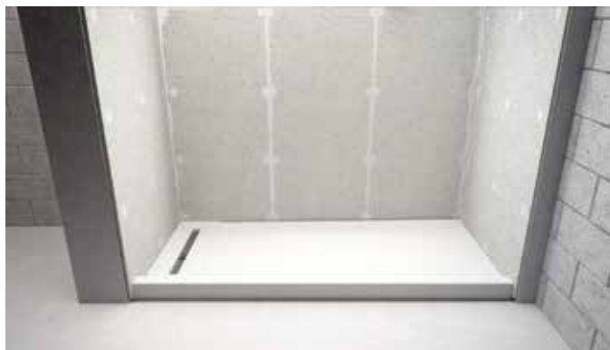
Figure 7: ShowerPerfect pre-sloped pans and drain support frame installed and ready for next step
