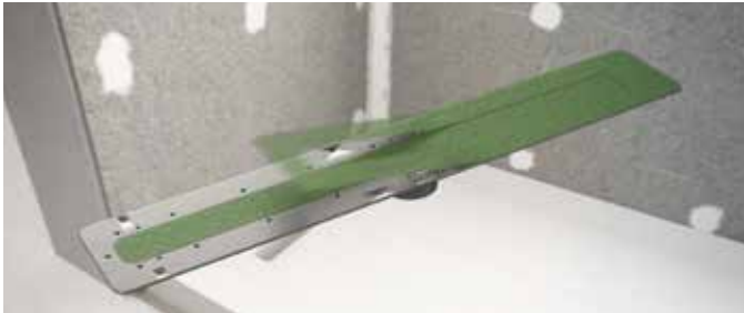
Figure 10: Peel off the green masking tape from the outer perimeter of the Linear Drain Body.
