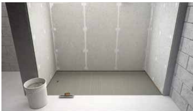
Figure 6: MAPEI's Ultraflex RS being used to set ShowerPerfect pre-sloped pan and drain support frame
